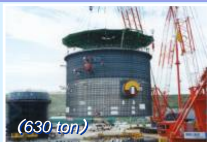
RCCV Lower Liner Module
